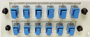
Patch Panel (12 Port Type)
